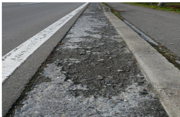
Fig. 1. Picture of a severely scaled waterway
